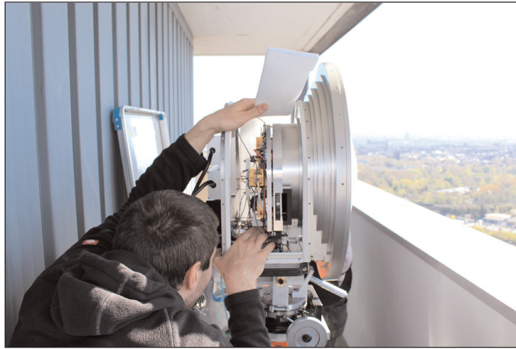
E-band transmitters with parabolic antenna.
