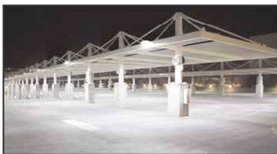
Bi-level LED lighting at parking lot of University of California, Davis.
