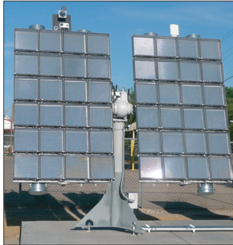
Semprius RDD system at TEP.
